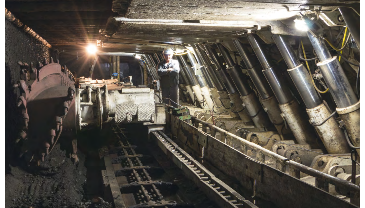
Hydraulic shield support with integrated chain conveyor and shearer
