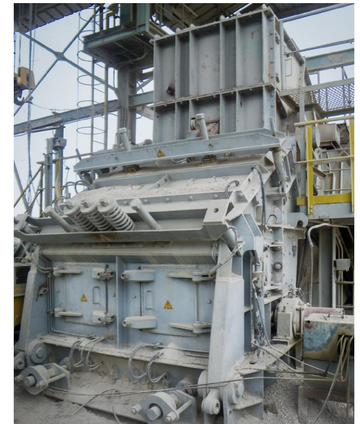
Limestone crusher in a cement plant
